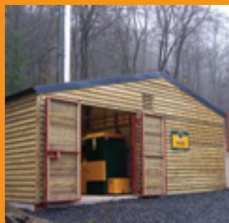
The boiler room is positioned 140 meters from the house.
