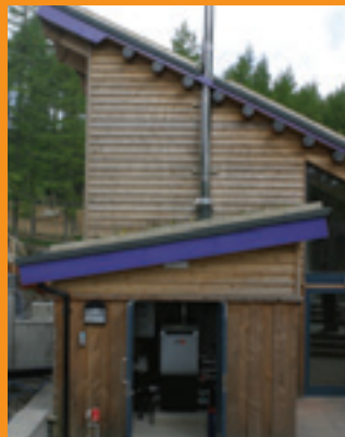
Compact boiler installation integrated with other sustainable technologies.
