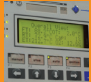
Constant monitoring of water temperature and flue emissions ensures maximum operating efficiency.
