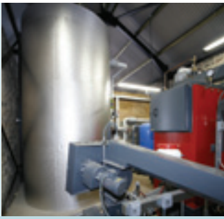
Fully automatic Binder boiler and high-volume accumulator tank.
