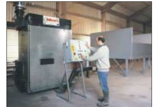
The Talbott's B3 boiler and feed hopper
