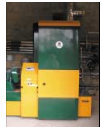
The KWB boiler system
