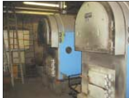
The converted boilers at Kirk Balk School
